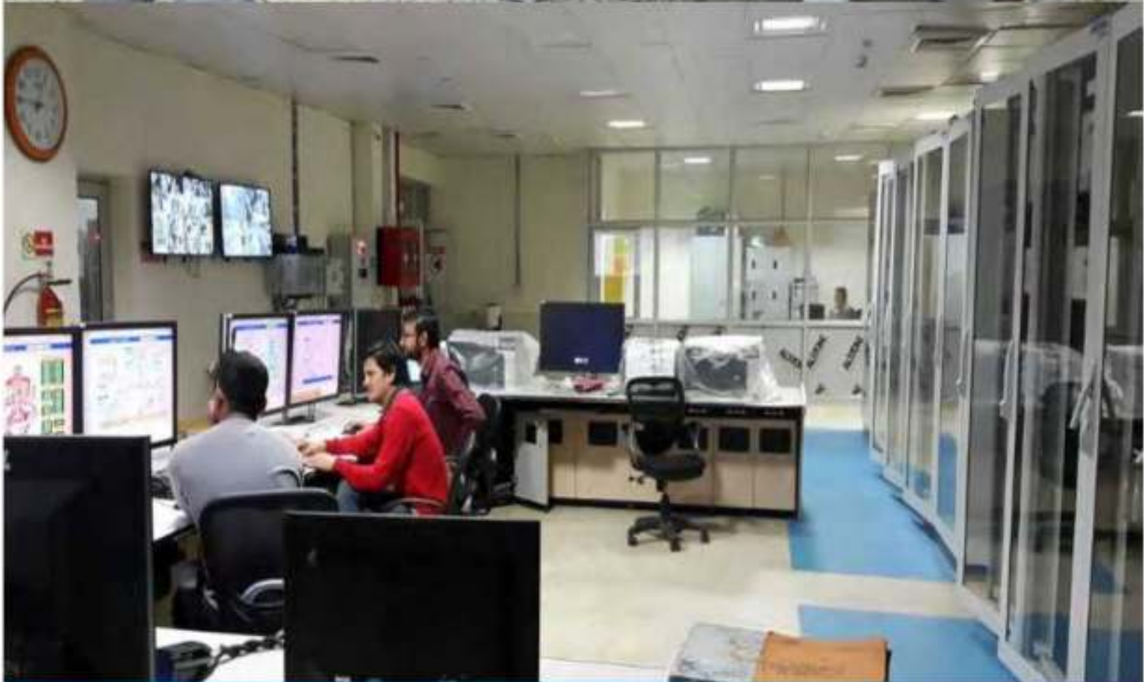
Power House Control Room Kashang HEP Stage - I
