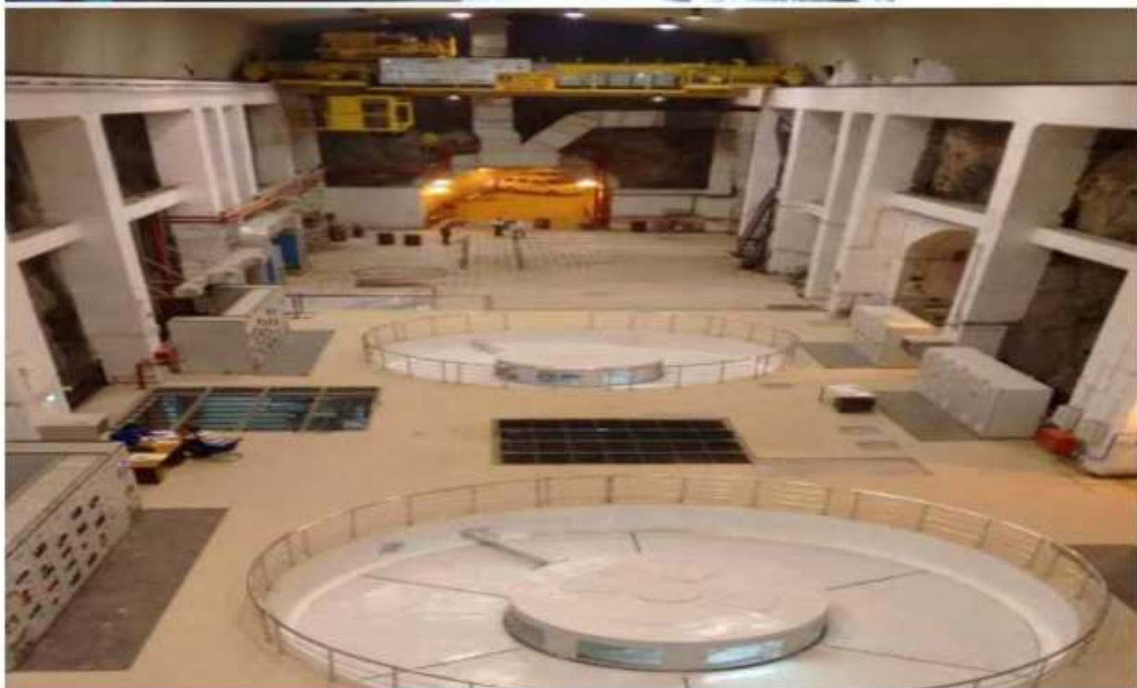
Machine Hall of Sainj HEP
