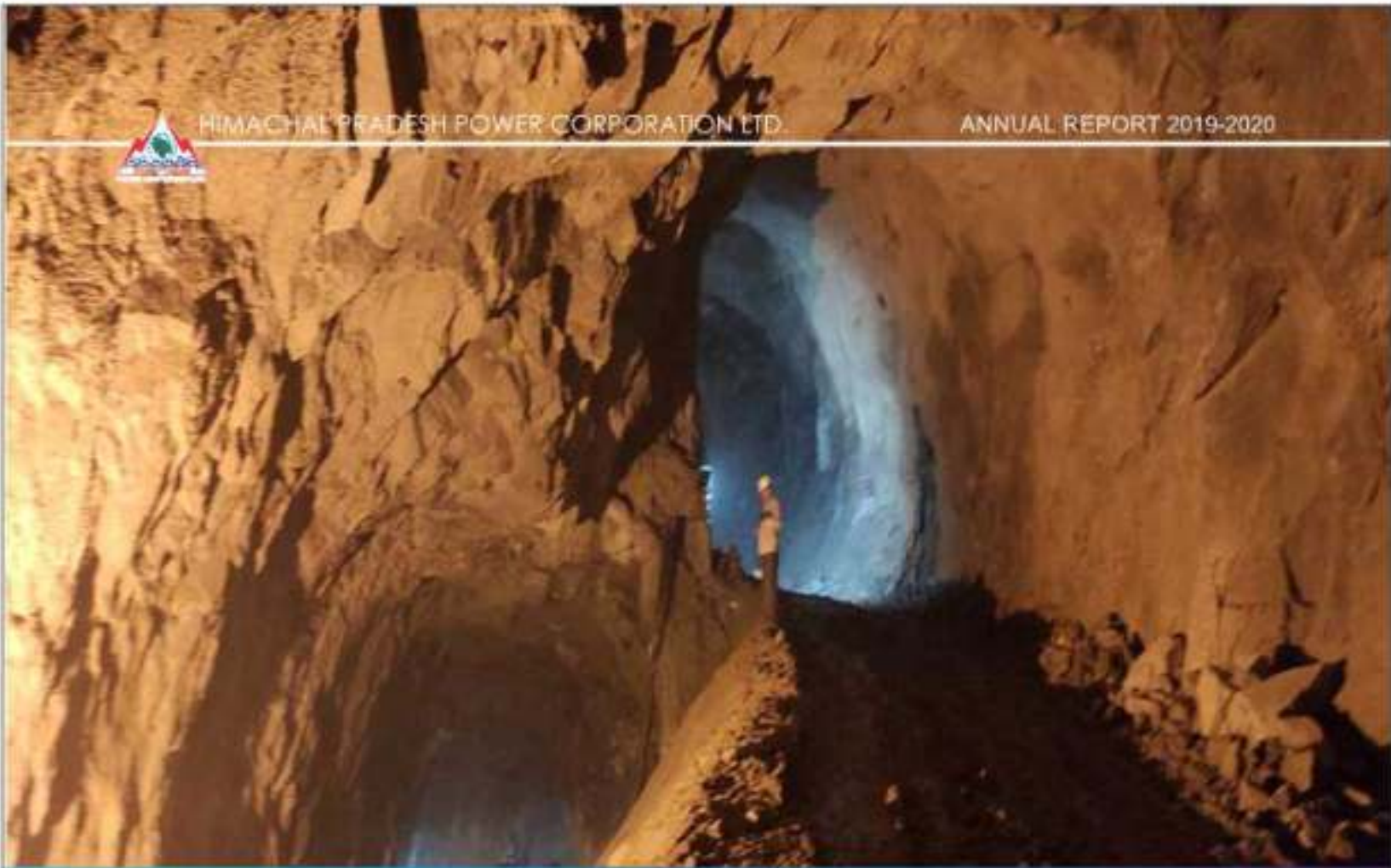
Butterfly Valve Chamber STK-HEP (450 MW)
